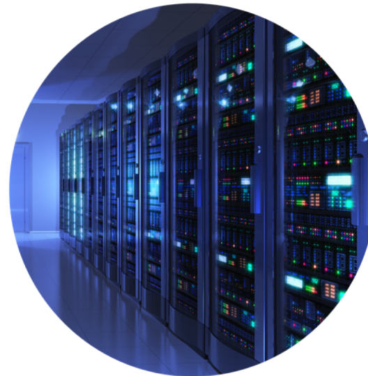
◀ Servers and networking ▶
